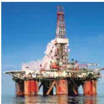
Corrosion protection of offshore structures requires robust technology.
