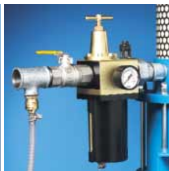
The maintenance unit is installed on the equipment.
